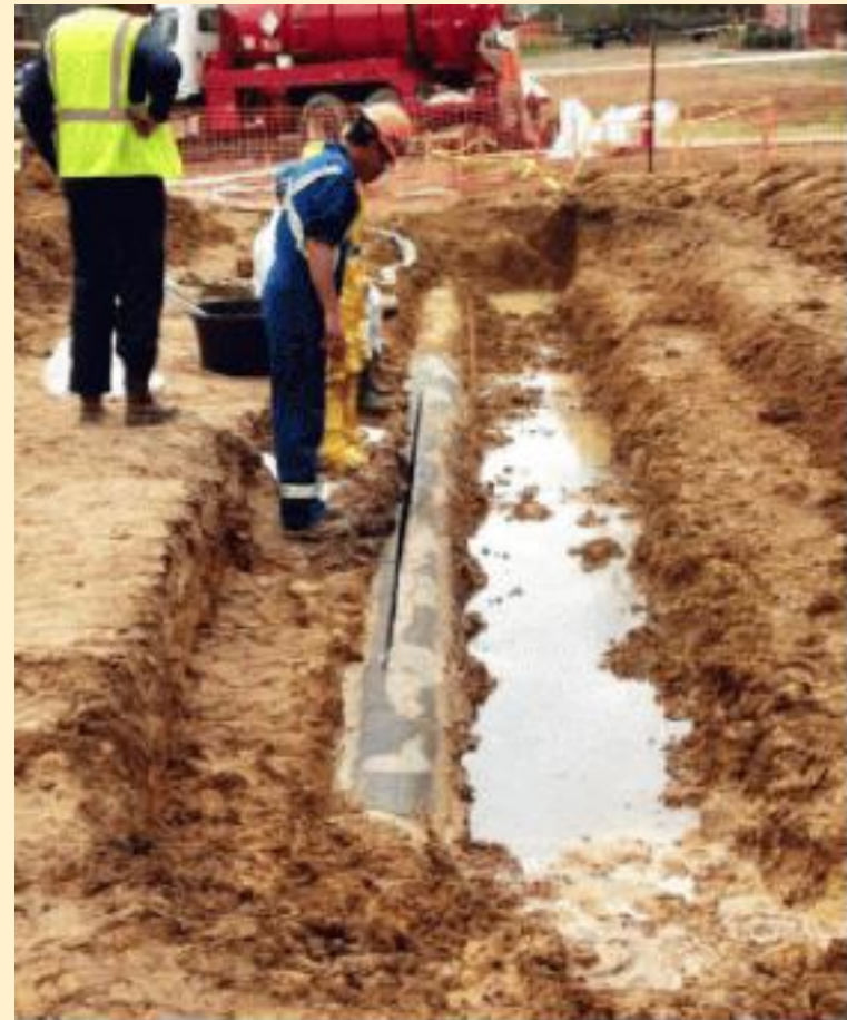
Exxon's Pegasus pipeline rupture/Credit: Duncan Firm
